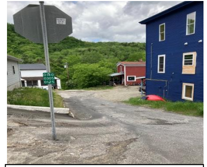
Intersection of South Main Street and Farr Street – after a minimal rain event.
