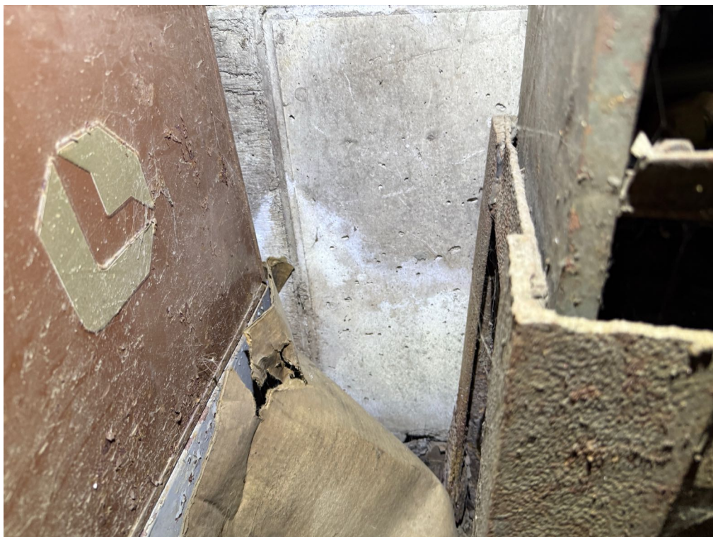
Figure 9: Efflorescence at West Foundation Wall
