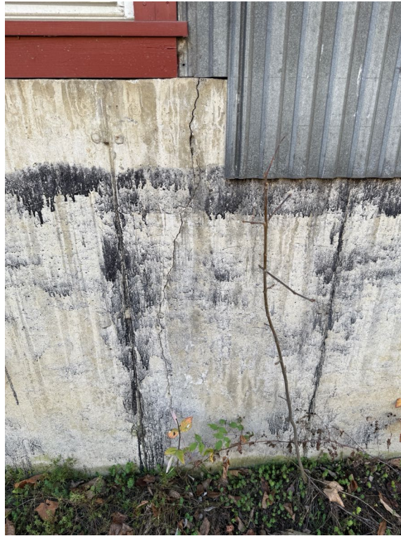
Figure 12: Vertical Cracking at Rear Foundation Wall
