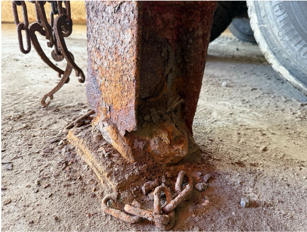
Figure 6: Steel Corrosion and Deterioration at Base of Interior Steel Column
