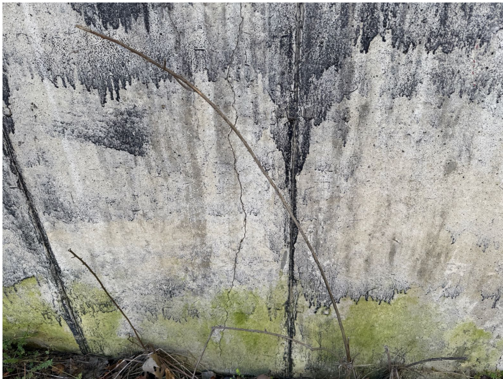
Figure 11: Vertical Cracking at Rear Foundation Wall
