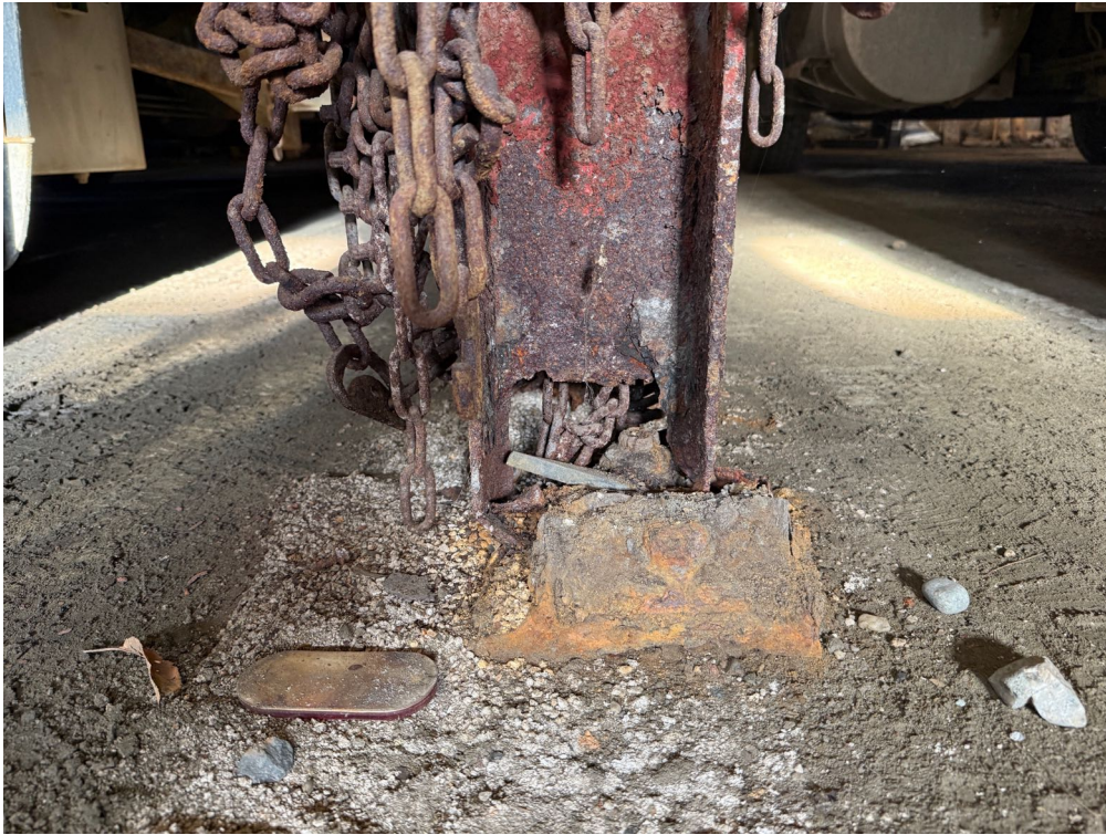
Figure 4: Steel Corrosion and Deterioration at Base of Interior Steel Column
