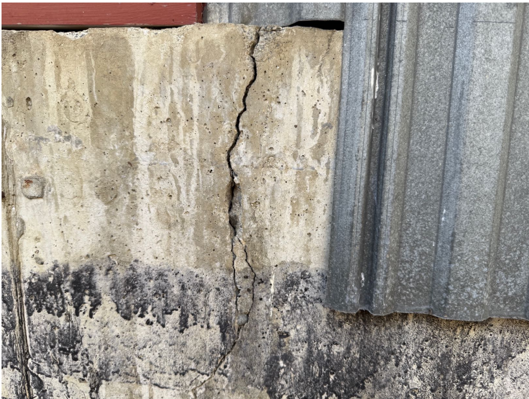
Figure 13: Vertical Cracking at Rear Foundation Wall
