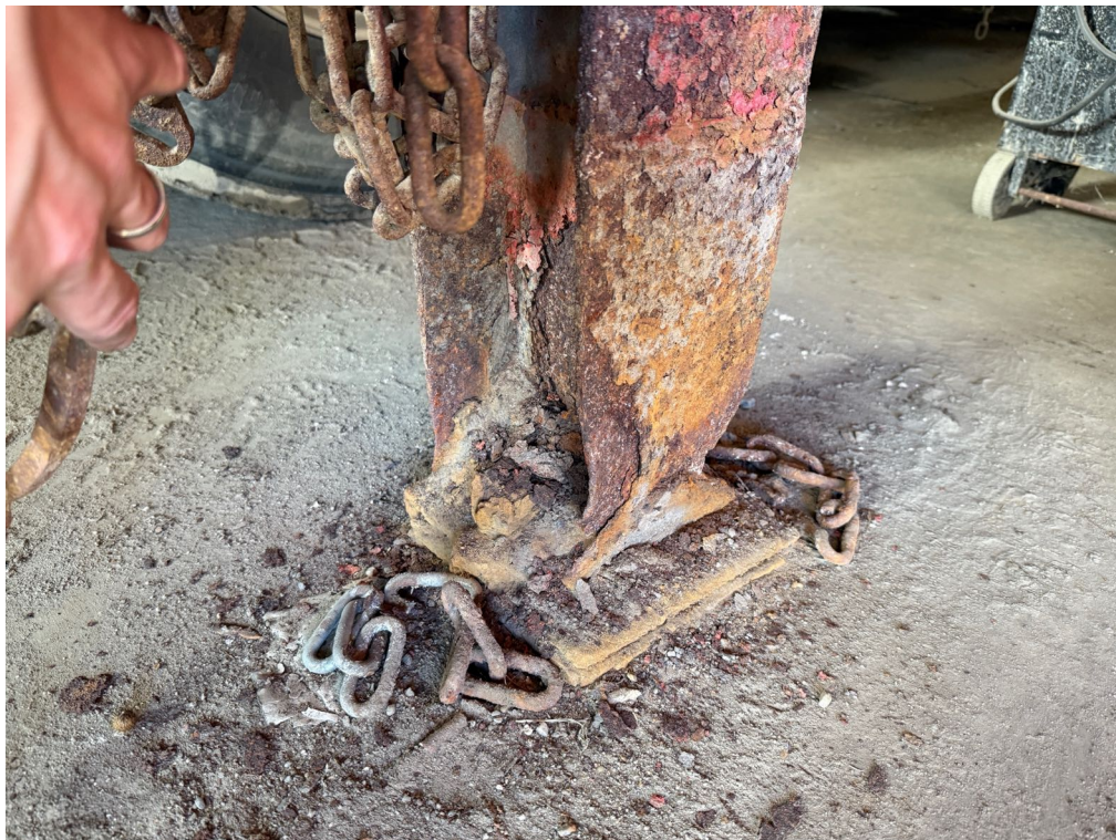
Figure 5: Steel Corrosion and Impact Warping at Base of Interior Steel Column
