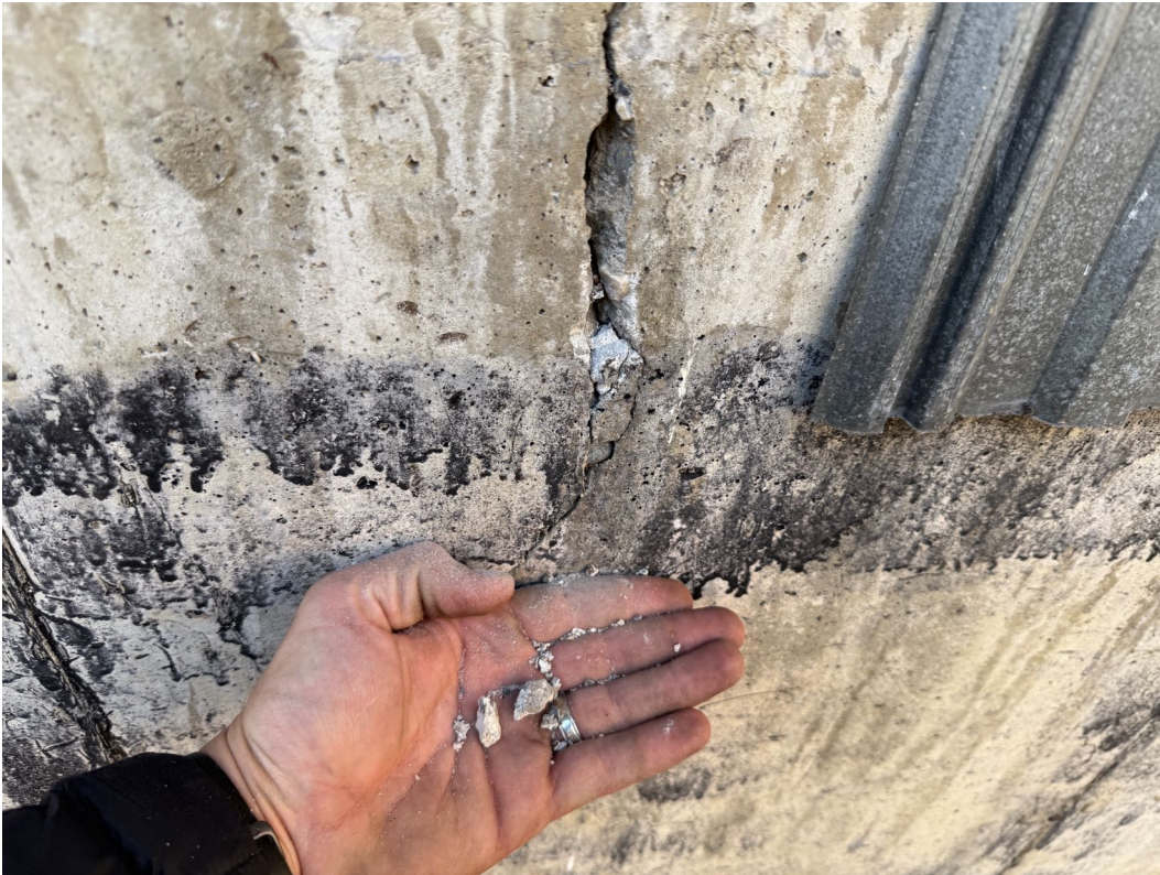
Figure 14: Vertical Cracking and Spalling at Rear Foundation Wall
