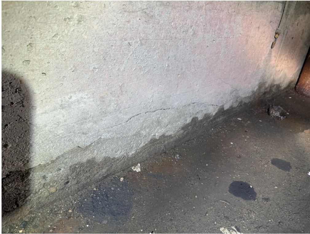
Figure 10: Active Moisture and Cracking at Rear Foundation Wall
