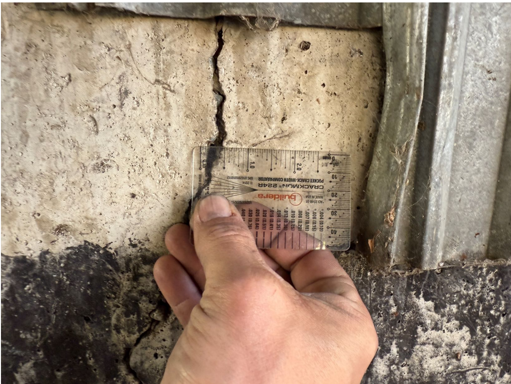
Figure 15: Vertical Crack Width Measurement (7/16\") at Rear Foundation Wall
