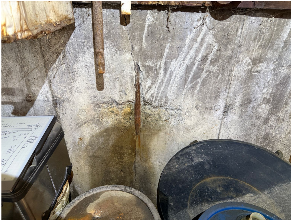
Figure 8: Spalled Concrete and Exposed/Corroding Reinforcing Steel at Rear Foundation Wall
