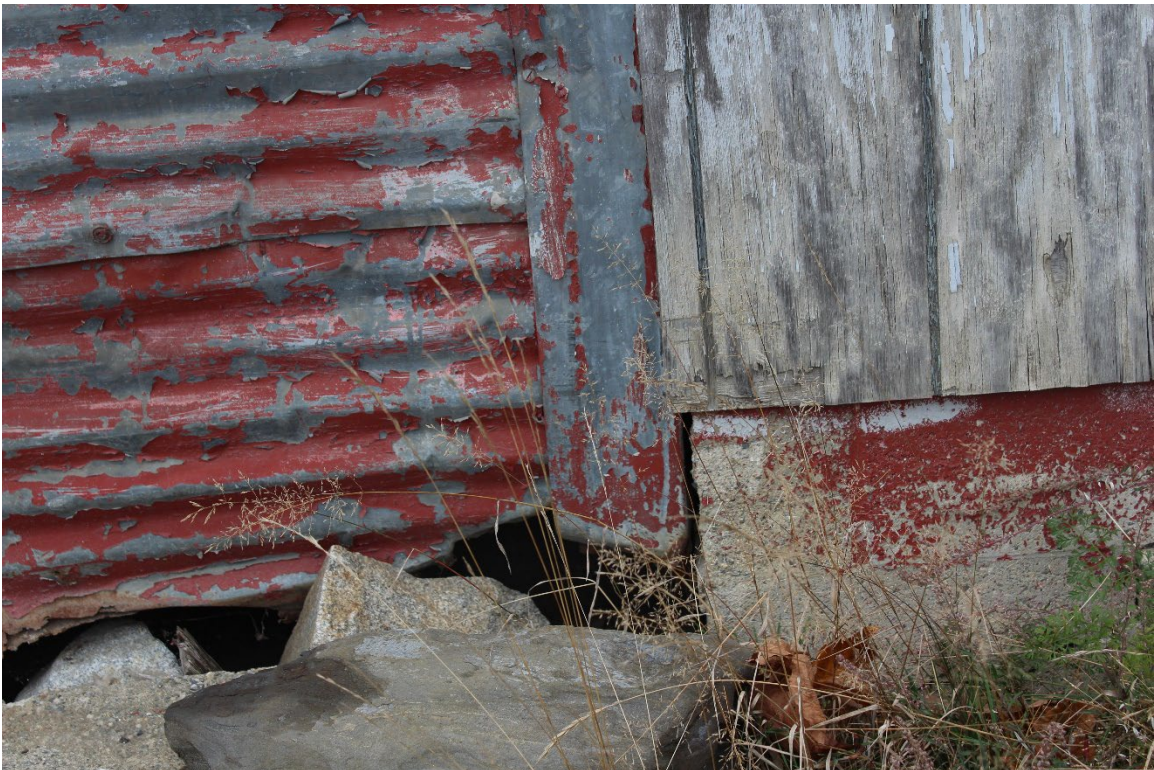
Photo 9. Two courses of concrete block were added to increase the height of the original poured concrete wall under the added, wooden stud-framed sections. Note that the original concrete wall is broken and heaved.
