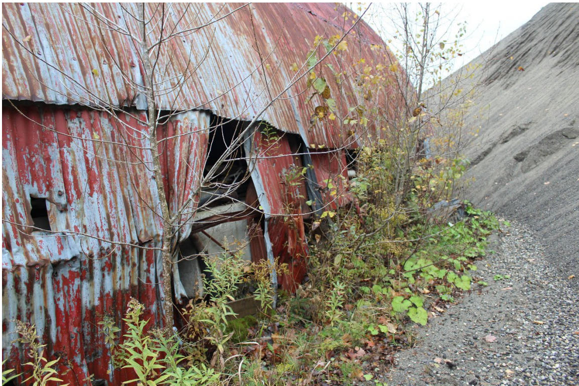
Photo 18. View SW, showing the unfortunate damaged west end of the north elevation.
