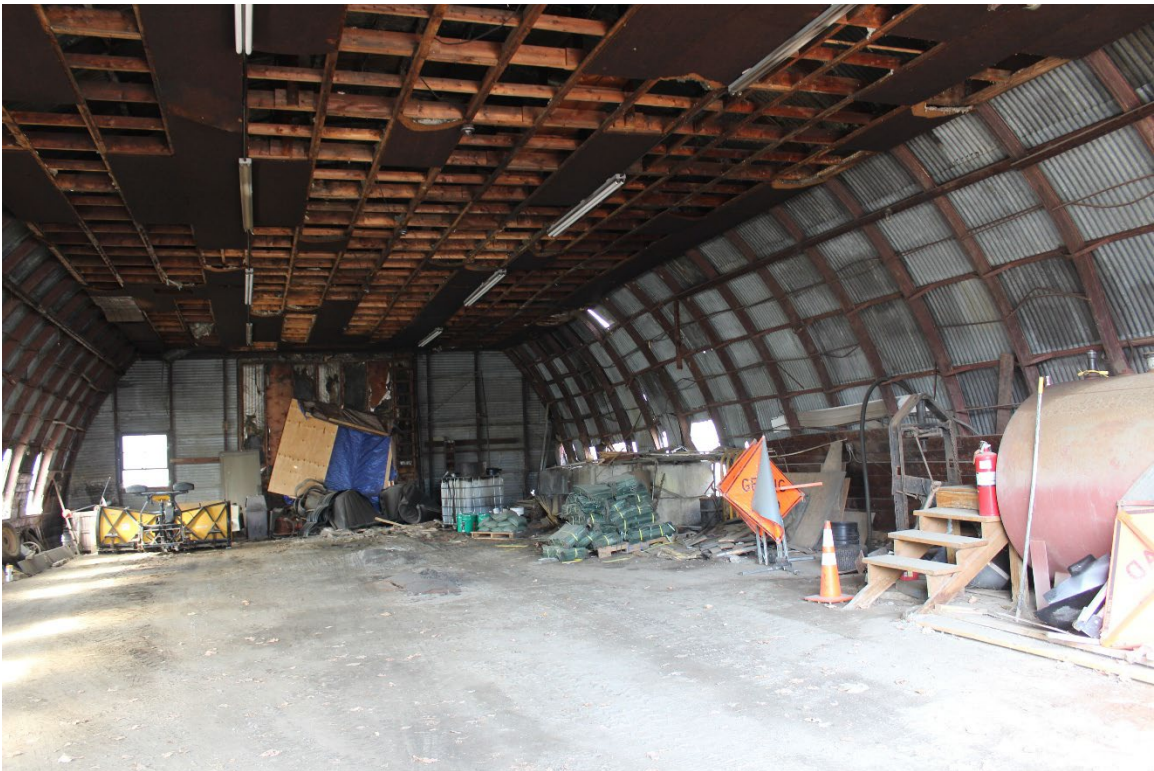
Photo 20. View NW, showing the metal stud-wall-framed west bulkhead and a portion of the arch-rib-framed north elevation. Some of the corrugated Sheathing and rib framing at the west end of the north elevation is damaged, broken or missing. An added wood frame suspended above the floor extends the length of the building and obscures the view of the upper third of the arched rib frame.
