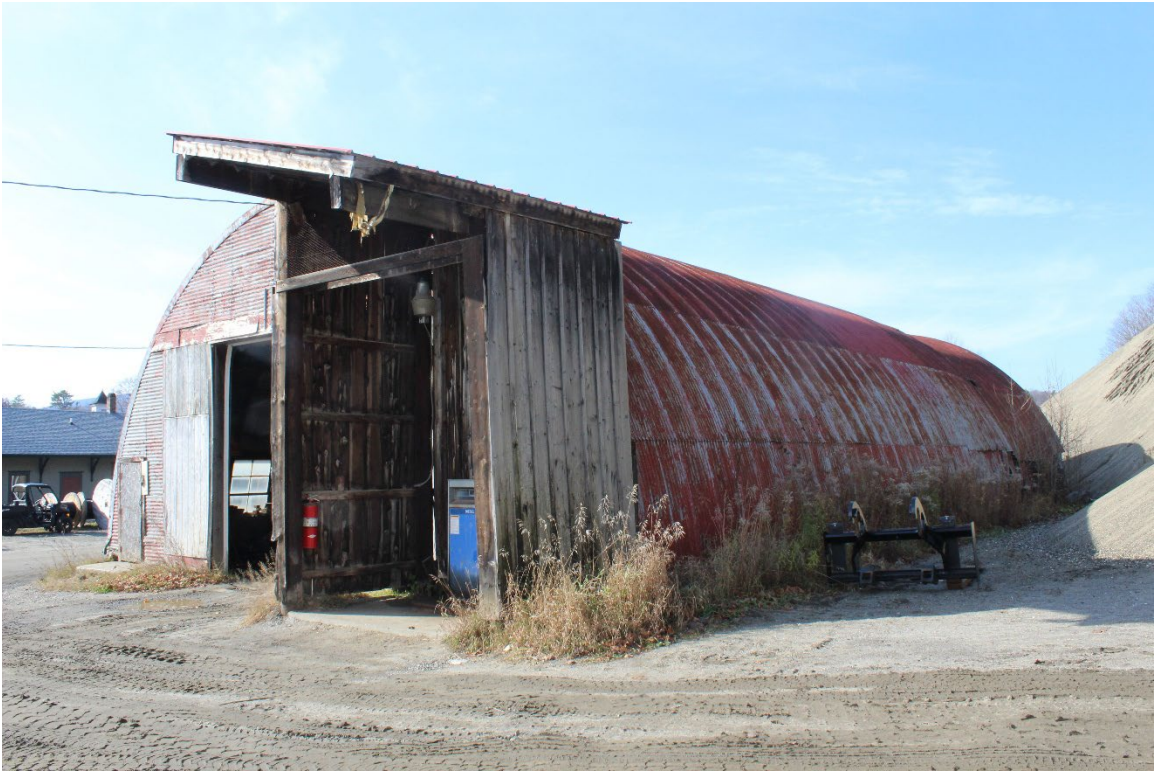
Photo 3. View SW, showing the solid north elevation. Some of the corrugated sheathing and associated framing at the west end of the elevation is bent and damaged, reportedly by road sand that had been piled against the building. The shed over the gas tank is not structurally attached to the Quonset Hut.
