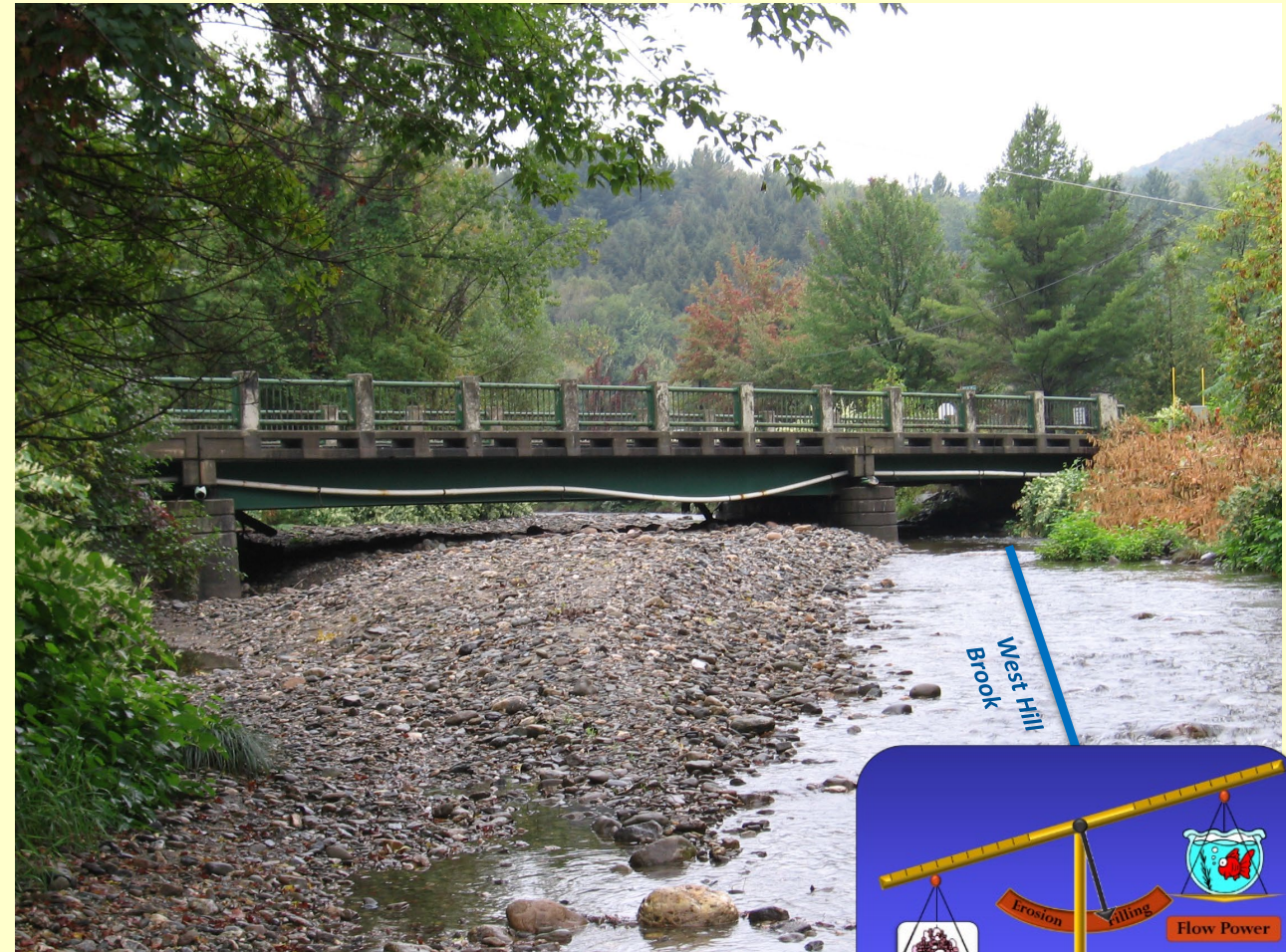
Downstream Face of the West Hill Road Bridge Sediment Buildup West Hill Brook Montgomery, VT . Image from DEC staff 2006
