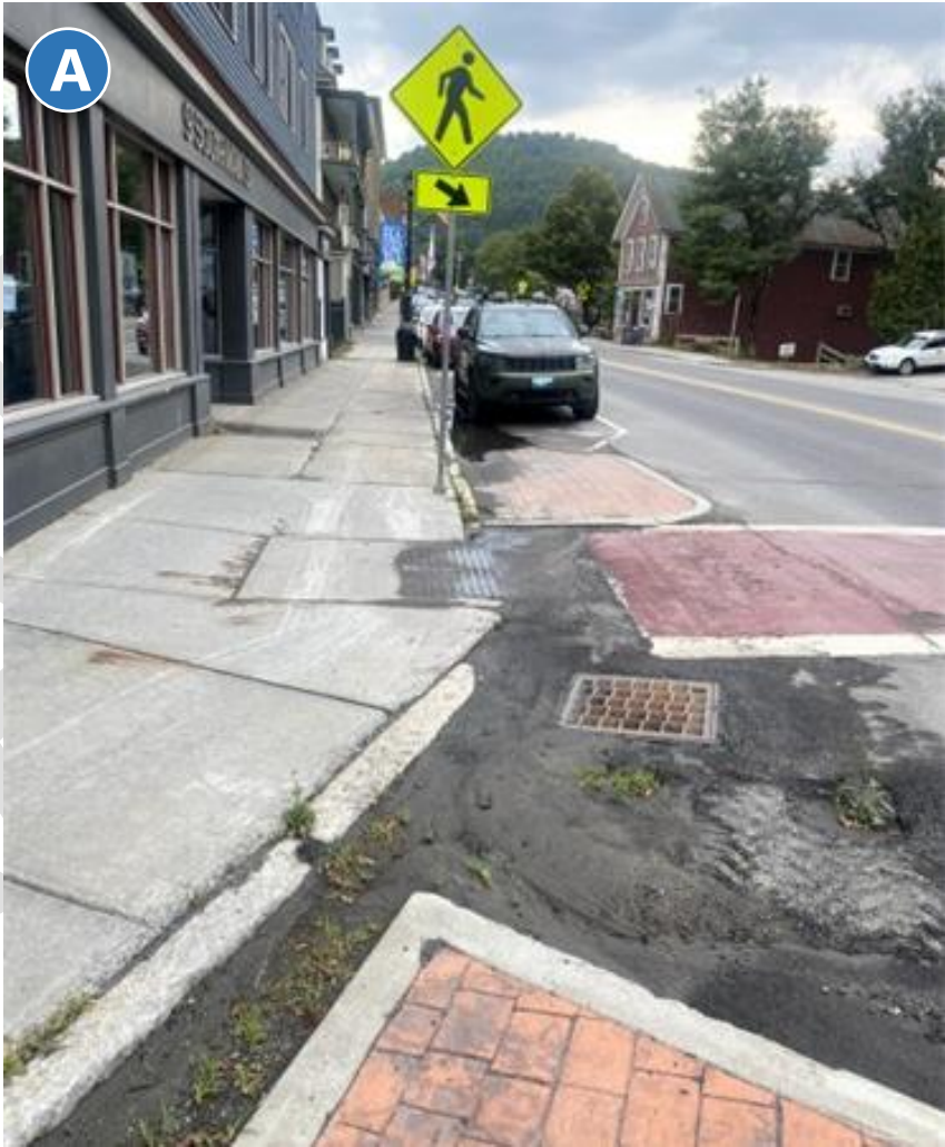
Figure 6 Sediment Accumulation in front of The Clip Joint
