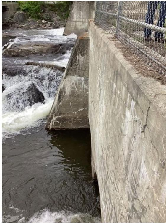
Effervescence and cracks above the two (2) 6-foot-diameter principal spillway outlet structure.
