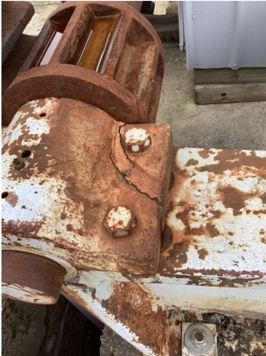
Crack observed in gate support.
