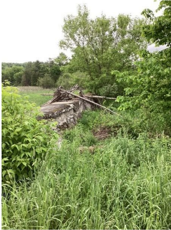
Example of concrete deterioration and delamination on the downstream face.
