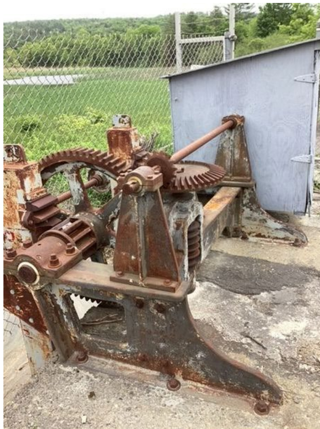
On left gate at the entrance of the spillway. Both gates are closed but are heavily leaking.
