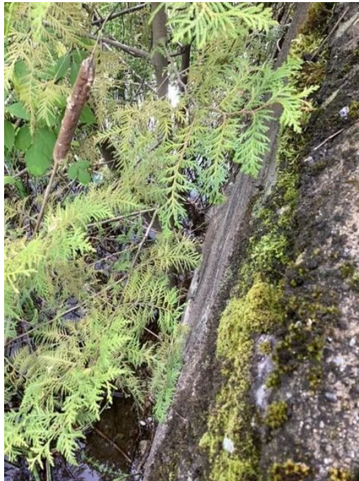
Tree growing out of upstream wall about 150 feet down left wall.
