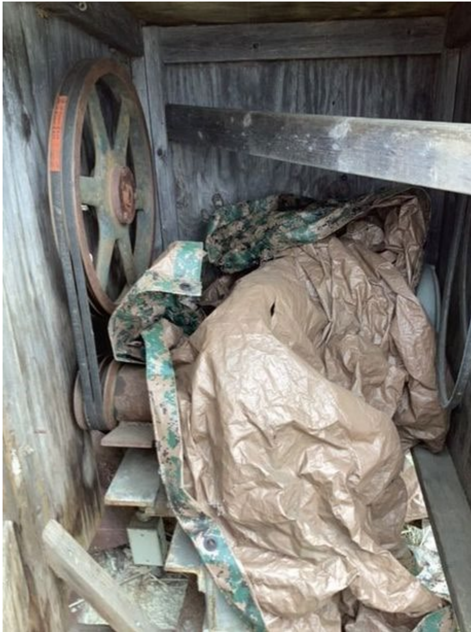
Inside of the housing where the gate operator is located for the left main gate.
