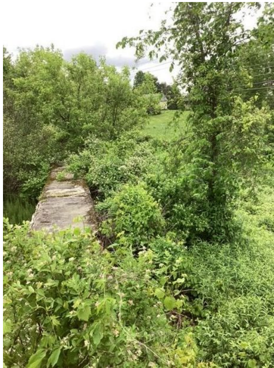
Vegetation obscuring downstream wall face.
