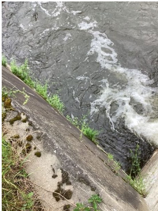
Bulging of the training wall on the left side of where the two (2) 6-foot-diameter principal spillway outlet barrels discharge.
