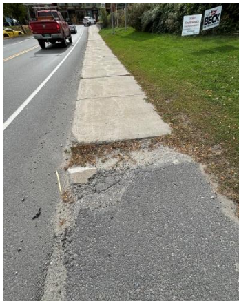
Sections have gaps and are crumbling.
