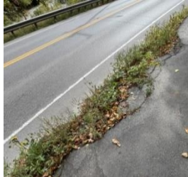
Cracked and crumbling sidewalk near large drop.
