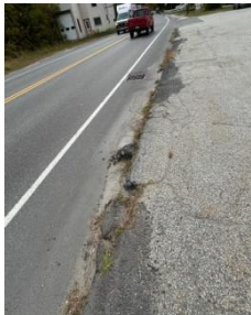
A slight curb cut is identified at Northeast Service Station.
