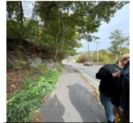
Vegetation overhangs the sidewalk.
