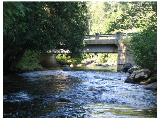
Figure 5. R30A. Bridge and channel constriction
