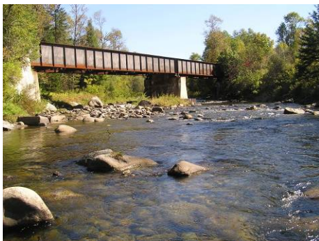
Figure 2. R26 Railroad bridge with mid-channel pier and aggradation
