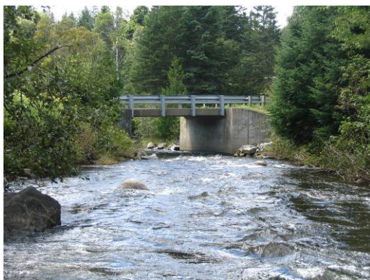
Figure 6. Undersized bridge with poor alignment in R30B
