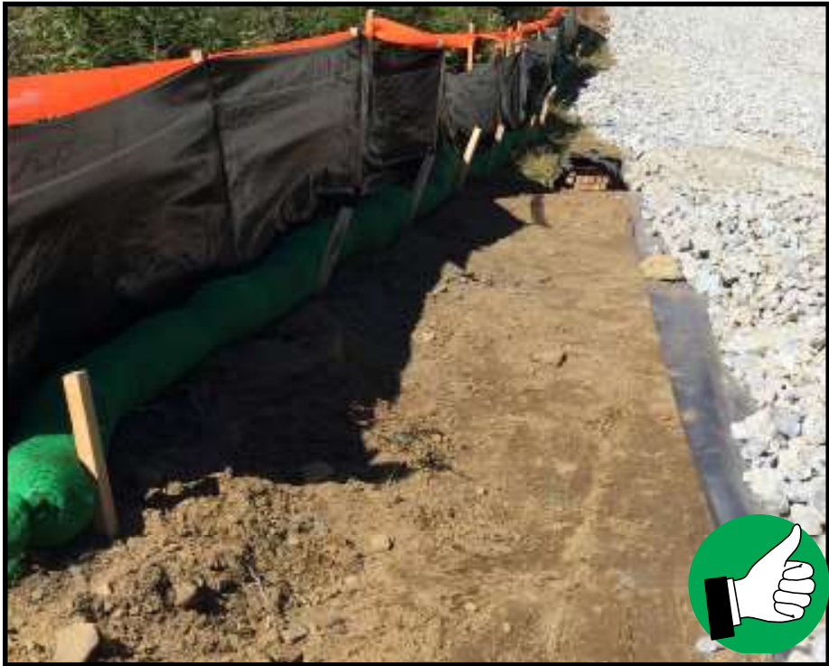
Use of a combination of silt fence and filter sock in place of reinforced silt fence for winter construction perimeter control requirements in proximity to a water resource area.
