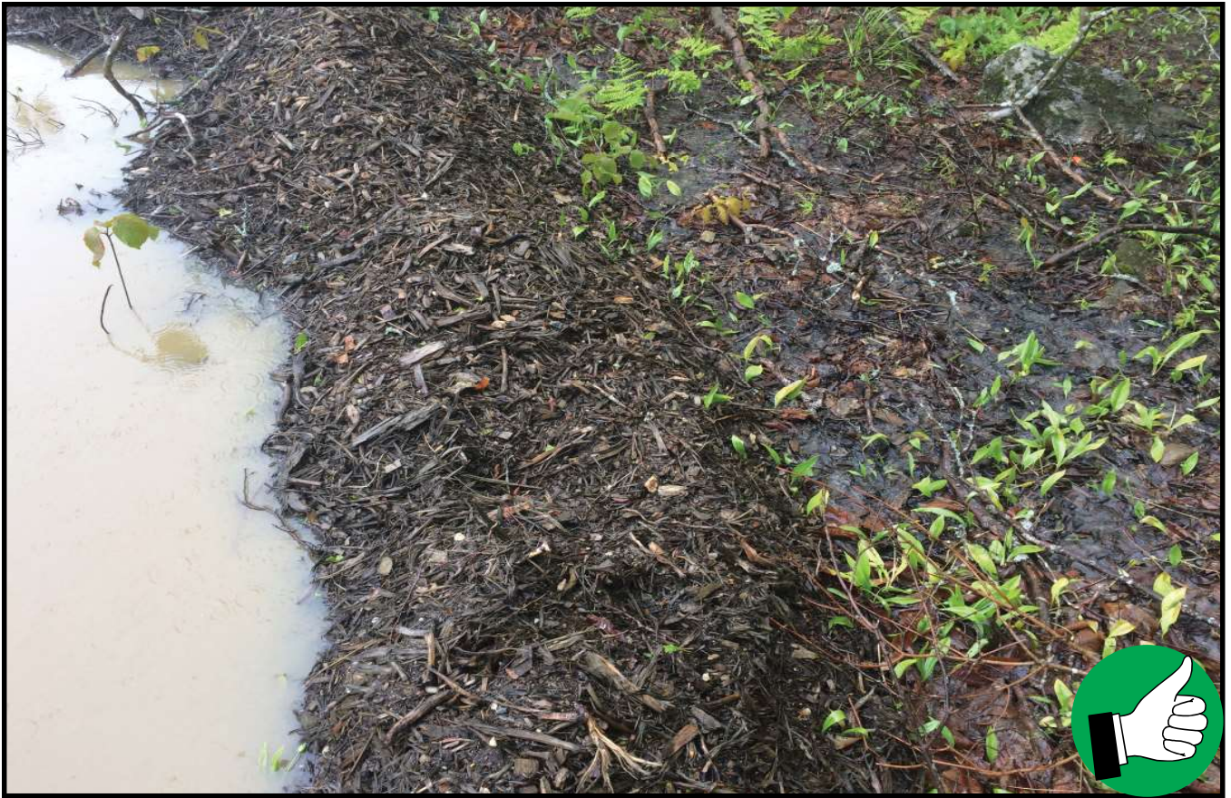
The erosion control berm above is allowing for both ponding and filtering of stormwater.
