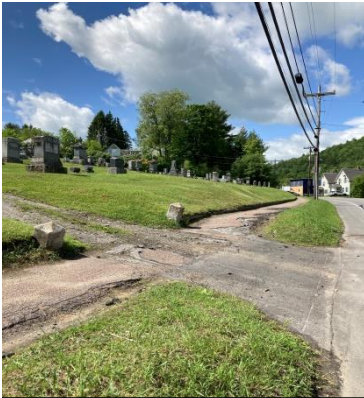
Sloping sidewalk on east side of South Main Street
