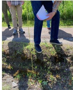
Curb erosion near the east sidewalk on South Main St.
