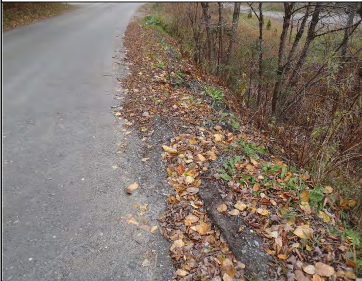
Photo 1. Shoulder berm/erosion and gully formation
