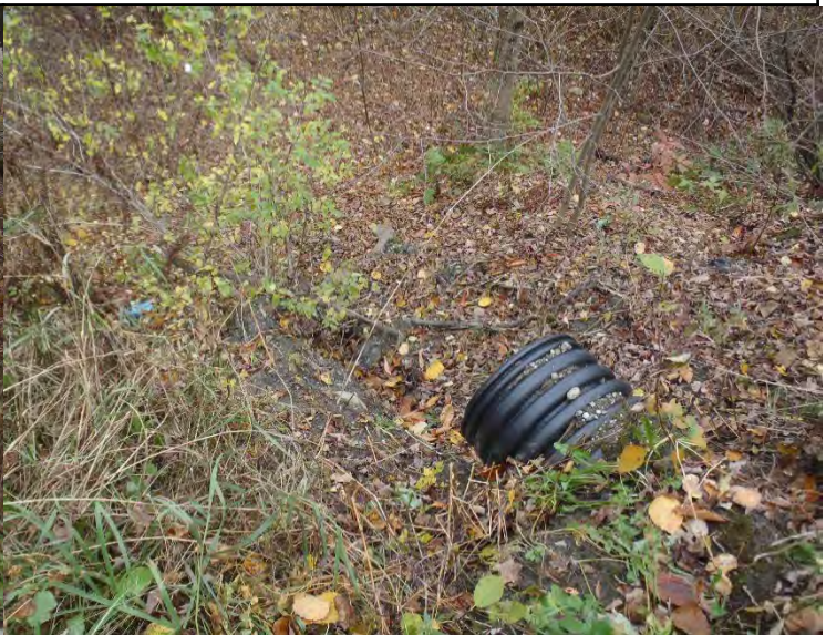
Photo 2. Elevated and eroding culvert outlet
