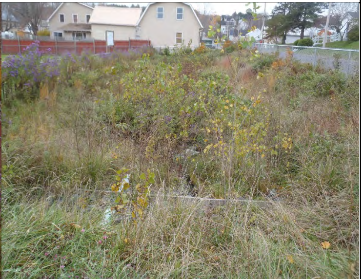
Photo 2. Bioretention area at Community Recreation Park in need of maintenance
