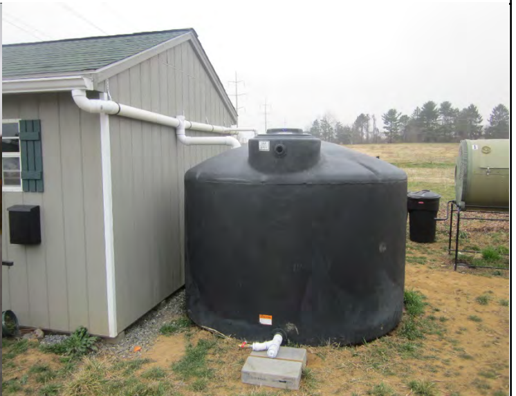
Photo 2. Example of a cistern used to collect roof runoff
