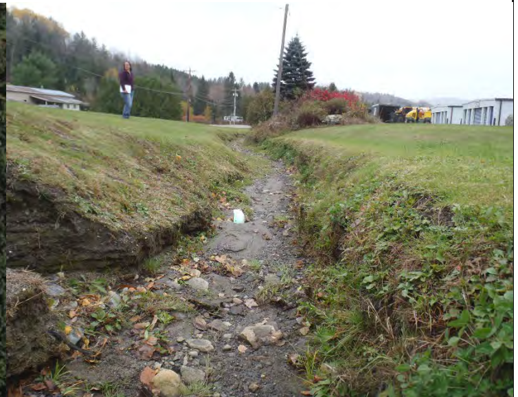
Photo 2. Erosion within drainage channel
