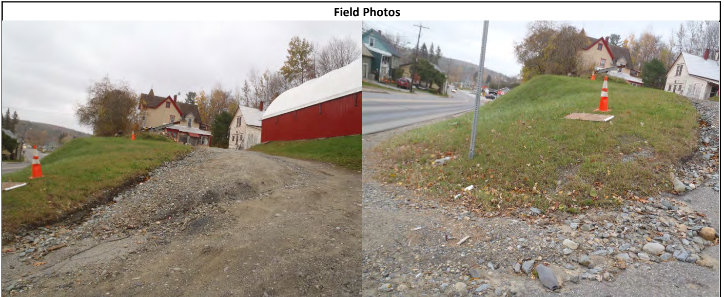
Photo 1. Driveway erosion at the home on the south corner of Hillside Street and Wolcott Street
