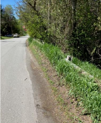
School Street embankment with dysfunctional guardrail
