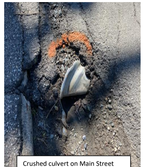
Crushed culvert on Main Street
