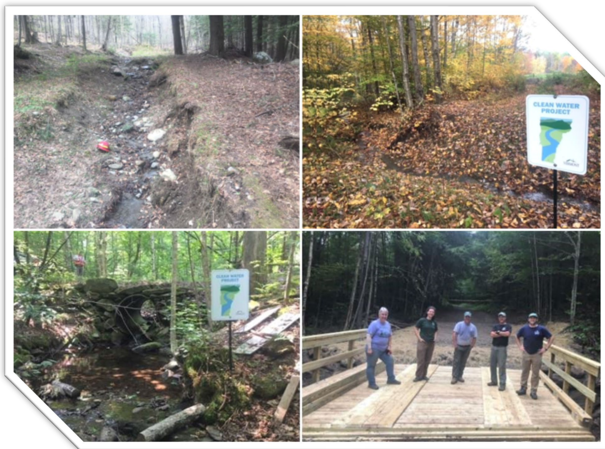
Figure 22. Upper photos left to right: eroded stream channel in Jacob Brook headwaters and stream channel restored. Lower photos left to right: undersized culvert over tributary to Waterman Brook and wooden bridge replacement over the tributary.
