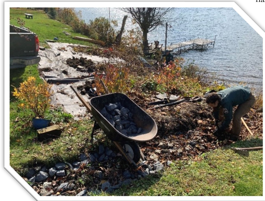
Figure 18. Vermont Youth Conservation Corps installing a no-mow buffer and stone-lined channel to infiltrate and slow runoff from impervious surfaces on the Lake Elmore shoreline (Photo by Peter Danforth).
