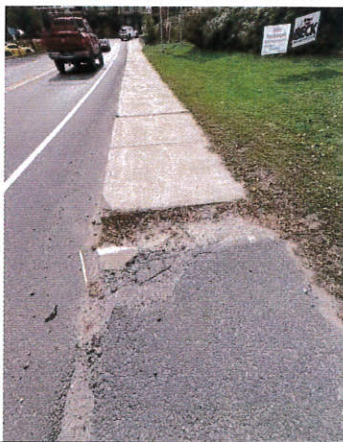
Sections have gaps and are crumbling.
