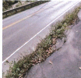
Cracked and crumbling sidewalk near large drop.
