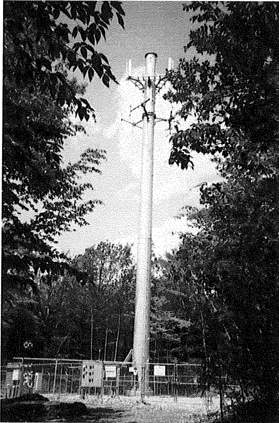
Westmoreland, NH Collocation Facility (100-foot Expandable Monopole)
